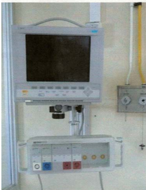
Wall mounted patient monitors were installed in the Cardiac Care Unit (CCU) and featured ECG, SpO2, NIBP, and IBP parameters.
